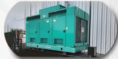
GENERATOR POWER BACKUP FOR COMMON AREA
